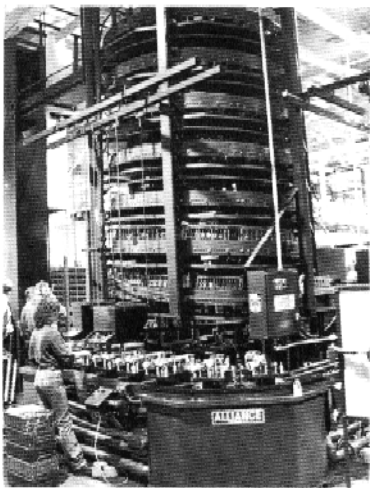
Spiral gravity storage units installed in the auto industry. These high capacity storage units automatically feed parts baskets to assembly lines. A reciprocating vertical lift loads the storage towers. These units can be ceiling supported to minimize floor space usage.
