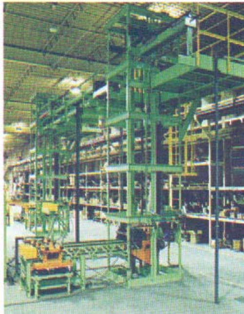
This conveyor transports engine blocks from the machining and inspection operation and lifts them over 14' to an overhead accumulation conveyor approximately 100' in length which crosses an aisle. The blocks are then lowered on demand from a second vertical conveyor to the floor, rotated 90 degrees and discharged to a wash unit.
