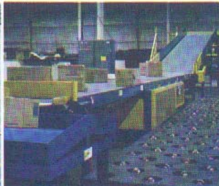
Belt conveyors are used extensively in the package handling industry. The conveyors are variable speed in either direction. Webb-Stiles expertise, with thousands of feet of package conveyor built and installed, makes it a leader in the industry.
