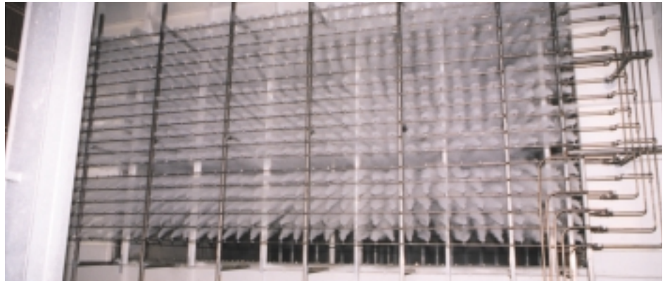
Gas Turbine Mist Cooling System
