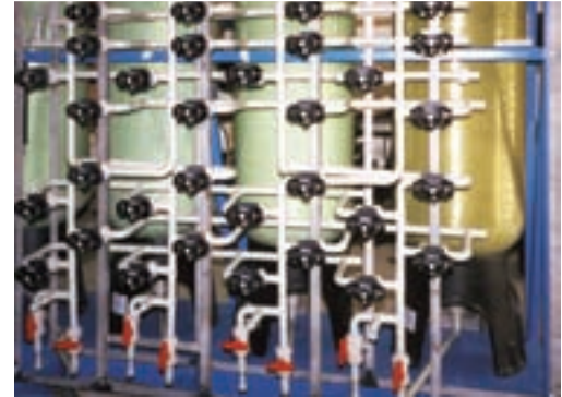
An installation of automated and manual Proline valves and piping.
