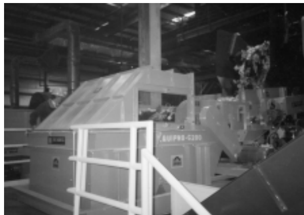
ECS-48" REO, Type HD with HV Pan Feeder Removing aluminum cans from municipal solid waste (MSW) at a material recovery facility.
